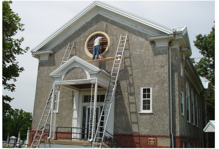
An expert from Glass Heritage LLC works on the church's oculus (round window) June 15. All 37 windows have now been restored.
